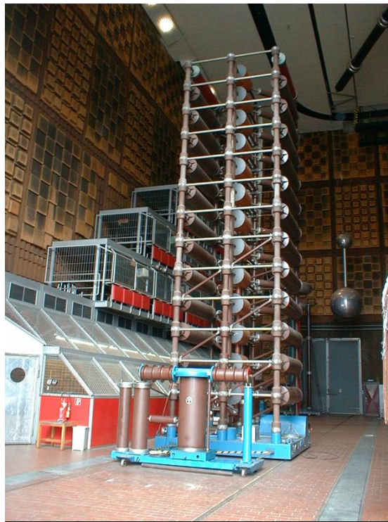
Photo 4: 3250 kV impulse generator, Graz University of Technology
