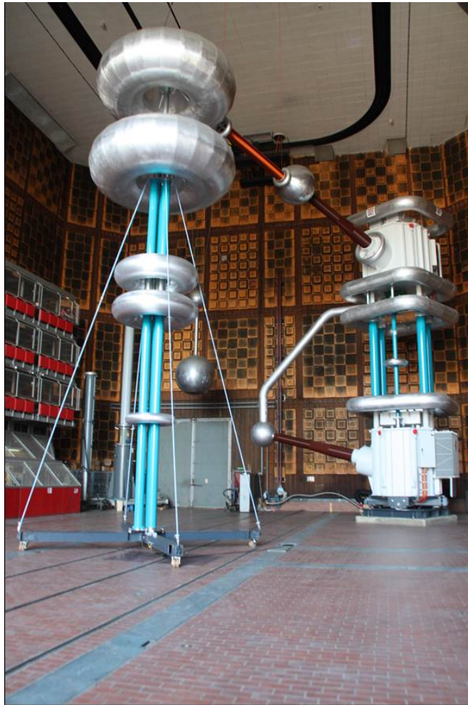
Photo 9: New 1500 kV AC generator in test position with the 1500 kV divider, Graz University of Technology
